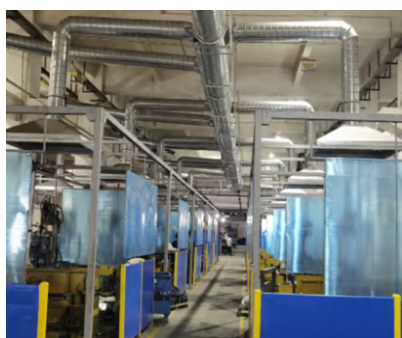
Newly installed weld fume and dust extraction system at an APG supplier
